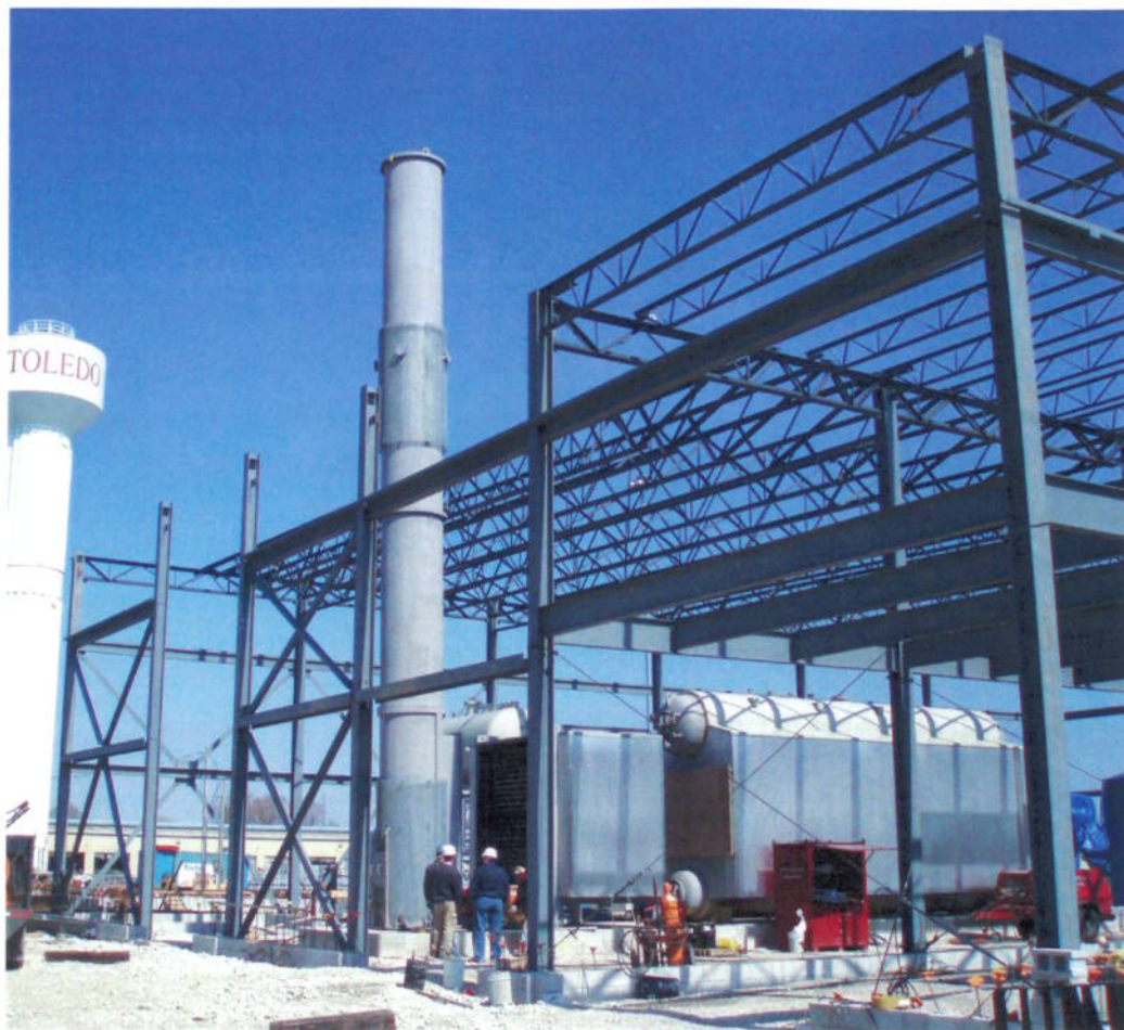
The cogeneration plant in Bay View involved three gas sources coming together to produce energy.
