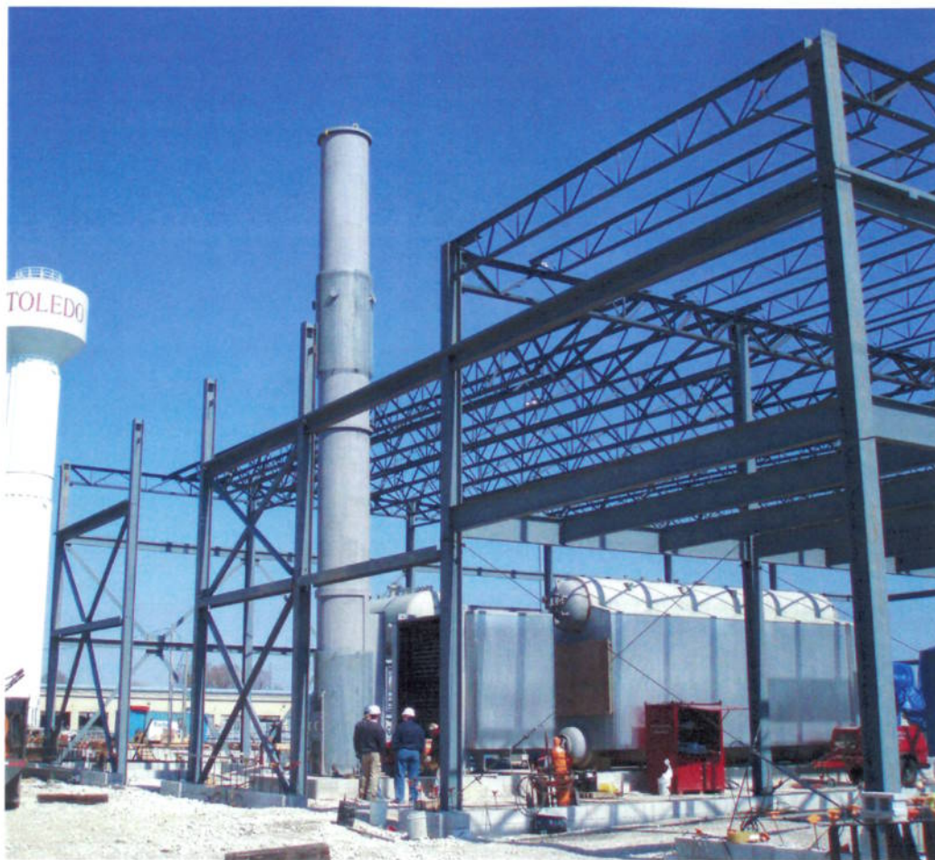
The cogeneration plant in Bay View involved three gas sources coming together to produce energy.
